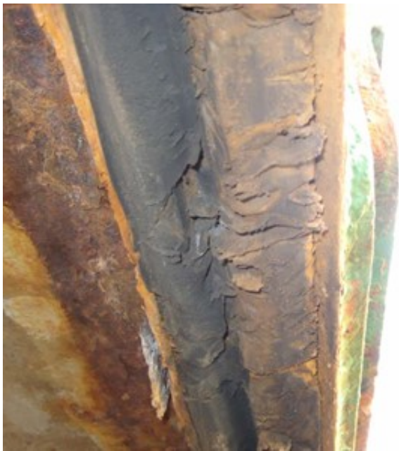
Figure 5: Hardened indented rubber seals
